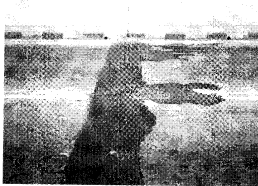
Figure 4 Flowing in asphaltic plug joint
