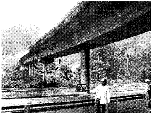
Figure 10 Water stain at the pier indicates leakage at joint
